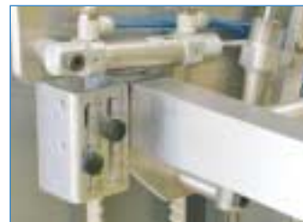
Limit switch assembly
